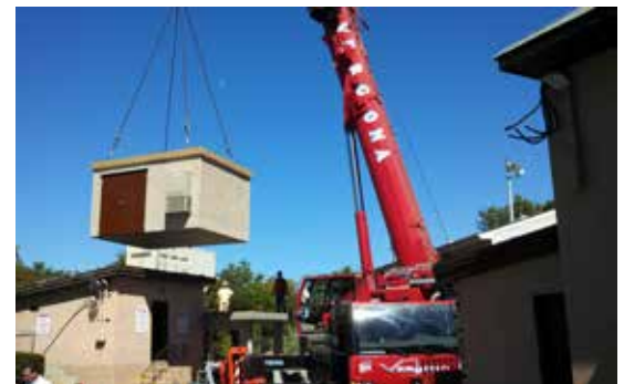
Flygt and Pumping Services provide turn-key solution
